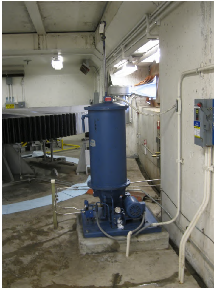
Figure 8-3. Automatic Grease-Dispensing System for Lock Machinery and Miter Gate Pintle
